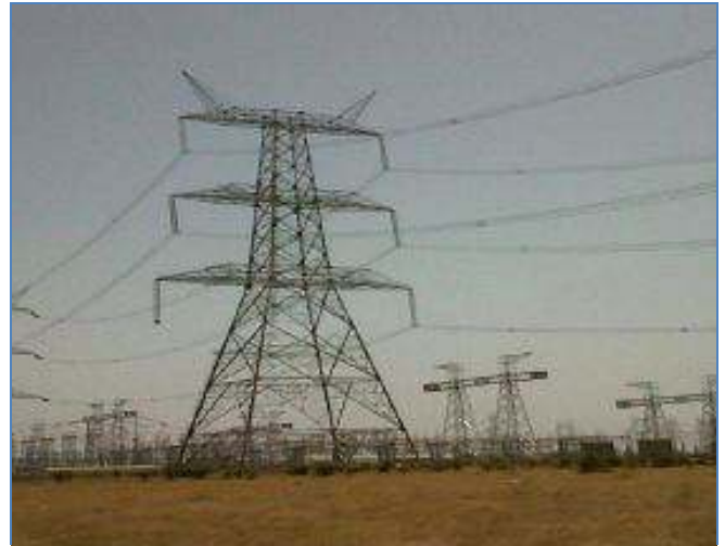
Fig. 3(b) : 1200kV Double circuit test line (D/C tower height: 125 m)
