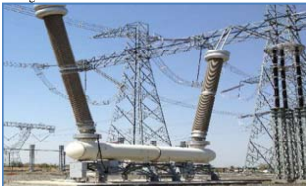
Fig. 1(c): 1200 kV Dead tank breaker
