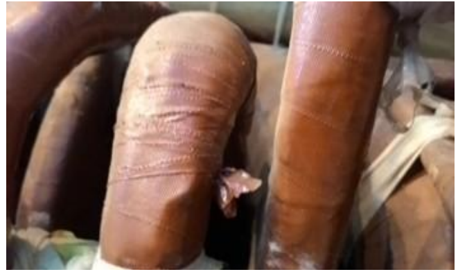
Fig. 1 : Presence of Knots, Lashes and Lower Air Gap between Phases
