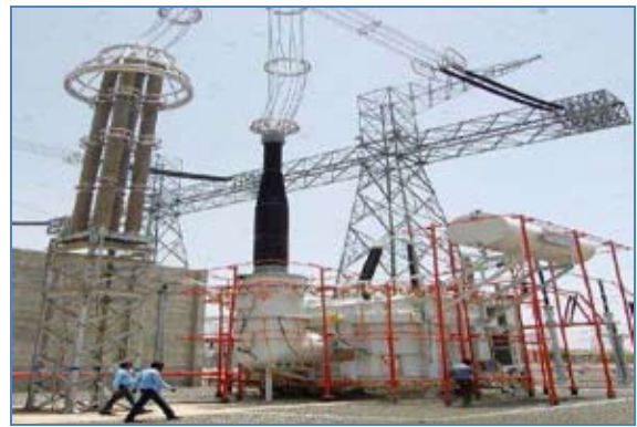
Figure 1(b): 1200 kV Multi-column surge arrestors
