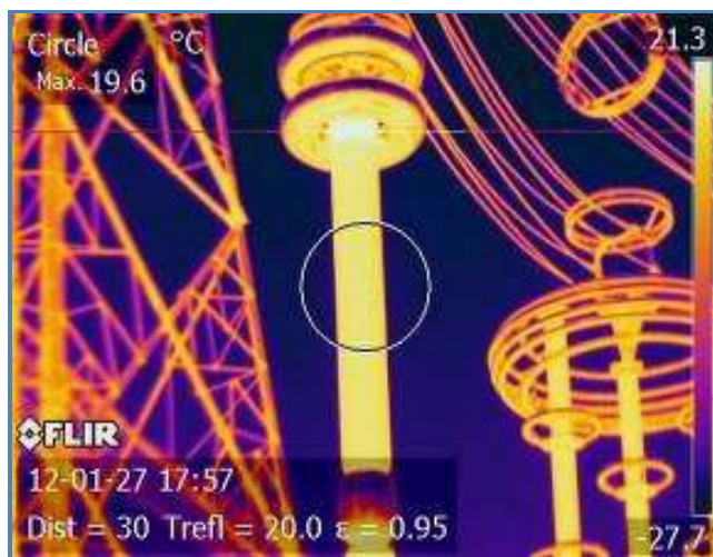
Fig. 8(c) : Thermograph image of 1200kV CB
