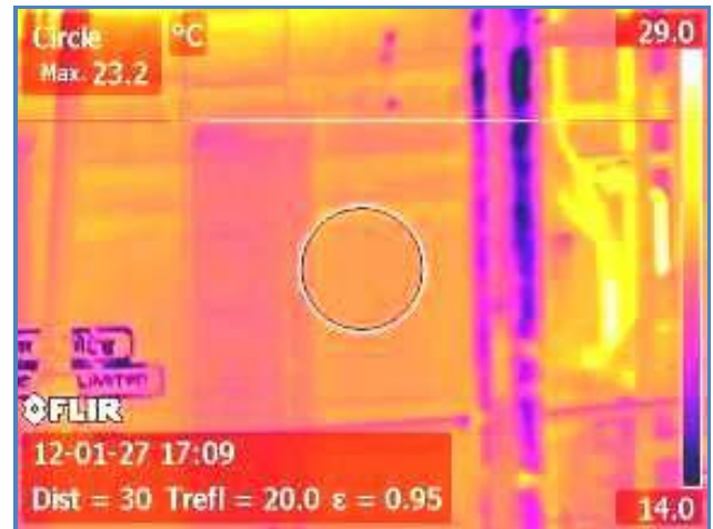
Fig. 8(b) : Thermograph image of the transformer body
